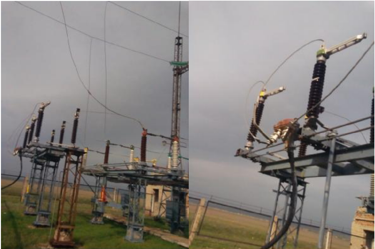
Figure 3 - Location of the ice melting plant at the substation
